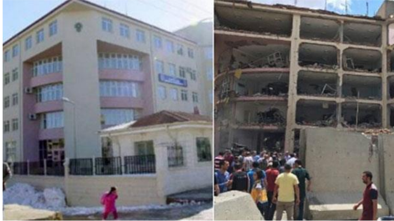
Figure 2. Collapsed infill walls of a State building in Turkey due to an intentional explosion (Yenisafak, 2016).
