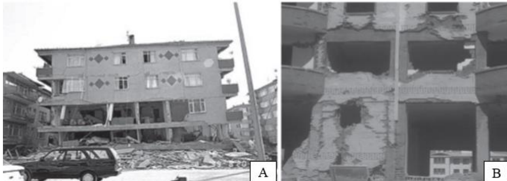
Figure 1. Out-of-plane failures of infill walls. (A) 1999 Kocaeli earthquake. (B) 2011 Van earthquake (Onat, Correia, Lourenço, & Koçak, 2018).
