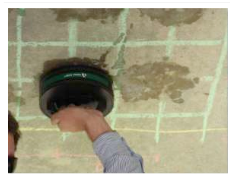
Figure 18. Corrosion Level Measurement with Icor equipment on the bottom surface of Prefabricated Slab
